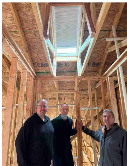
L-R: Steve Bushnik, Anders Dam Vestergaard and Tim O'Neill in an upstairs bathroom in a T&M home under construction in Glastonbury.
