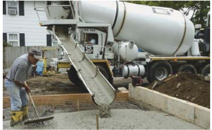
Pouring the basement floor O&G concrete with recycled glass for added strength. Wire mesh and spray foam over the trap rock for insulation.
